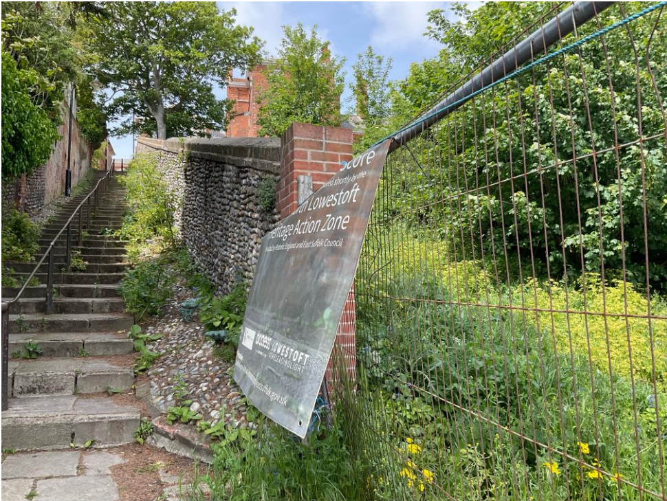
Figure 4: Own photo of Crown Score today (2023), in need of love and attention; also showing derelict land alongside with owner unknown (once a ‘hanging garden’ and could be again).
