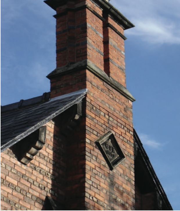
Figure 3. The gable and chimneystack of Edward and Sophia Kemp's house at 74 Park Road West, Birkenhead, with the datestone. Photo: author
