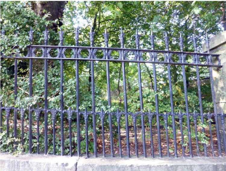
Figure 6. Doune Terrace – a short section of the original railing survives and could be closely copied to supply the missing length, c.1820
